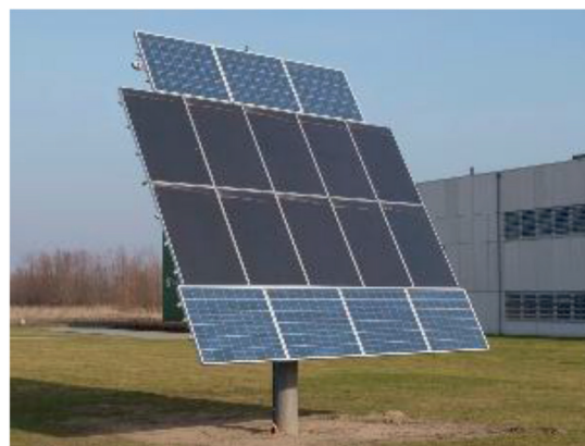
Fig. 54: Solar tracking system at Greenbridge (argus powermonitor.be)
