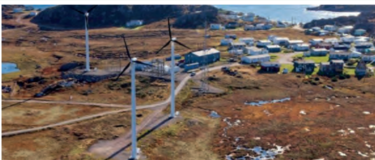
Afb. 63: SkyGrid Energy microgrid - North Kohala, Hawaii
